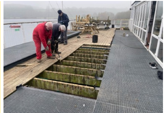
A few of the decking team at work - thanks to all who contributed to the 220 hours of time it took to make the decking much safer.
